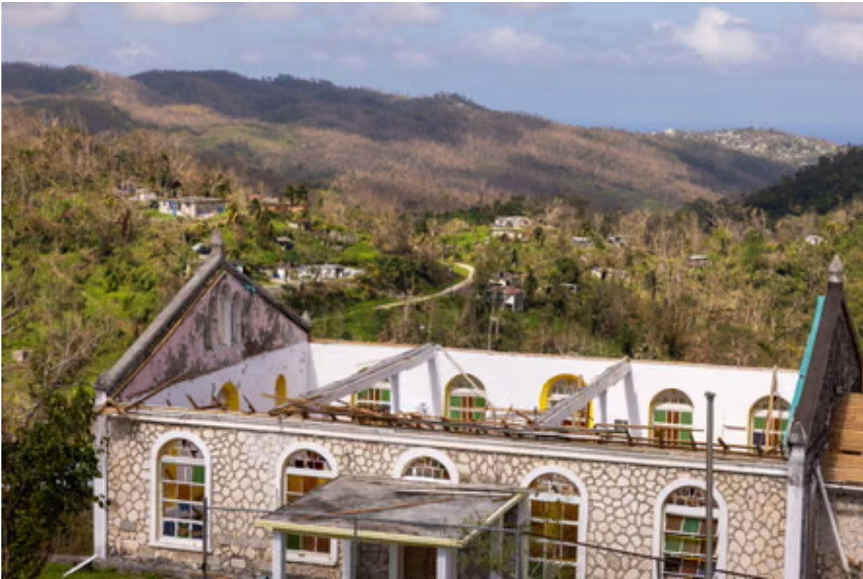
📷 Mount Gurney church demolished by the passage of Hurricane Melissa.
